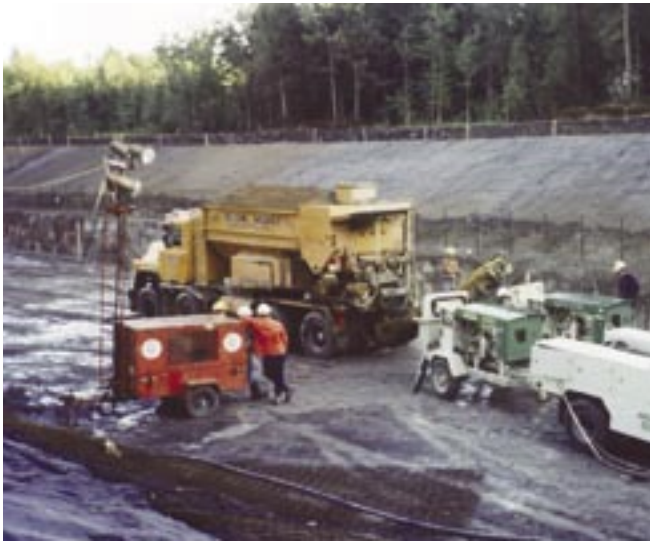
Fig. 5: Concrete mobile mixer supplying shotcrete for two pumps for access ramps on Grondines Tunnel under St. Lawrence River, Lotbinière, QC
