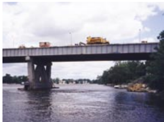
Fig. 3: Dry-mix shotcrete supplied with concrete mobile mixer for pier repairs of bridge over Rivière-des-Prairies River, Montréal, QC
