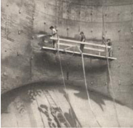
Restored, reinforced gunite flue at American Smelting and Refining Co., Helena, Montana, 1924
